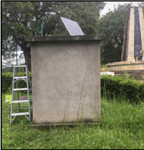
Figura 27: panel solar instalado
